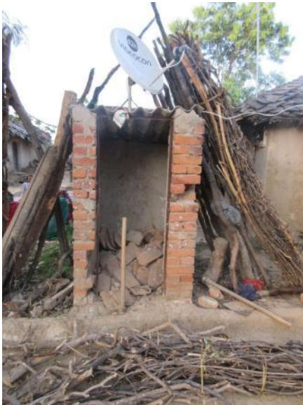
Incomplete and unused toilet
